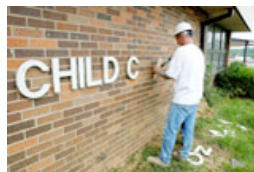
Bill Cain with Konzeny-Wagner Construction removes the sign from the Ferguson-Florissant School District's child care center on Brotherton Lane in Ferguson. Construction began June 9 for the district's new Challenger Learning Center inside the building. When completed, the center will feature space flight simulations and a mission control center modeled after NASA's Johnson Space Center. (Michael Reigner photo/Suburban Journals)
